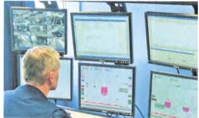
Kiosk/touch-screen operator consoles
